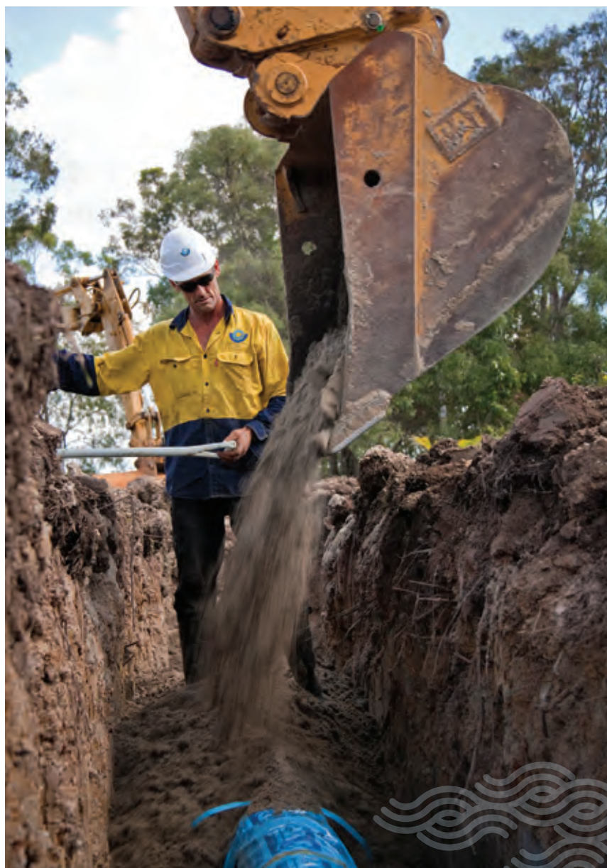
Logan Water Alliance's construction contractors install a new water pipeline using an open trench construction method.
