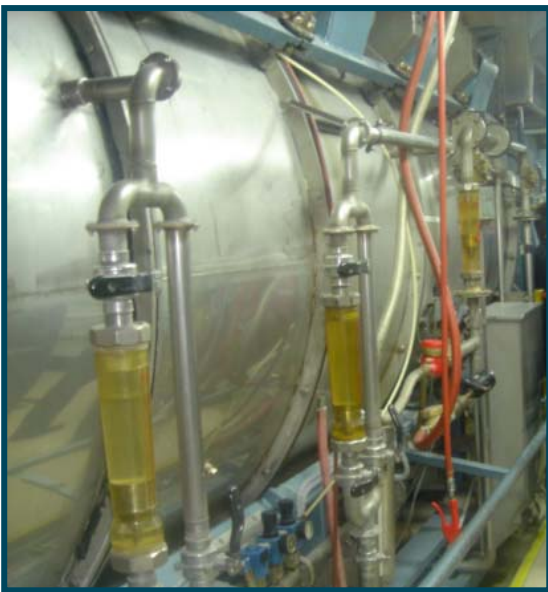
Intricate water efficient technology at Jupiters Hotel and Casino
